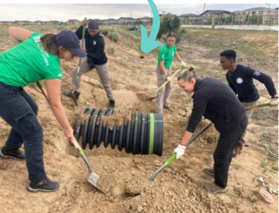
Mile High Youth Corps & NR Intern bury a tunnel to build coyote dens.
